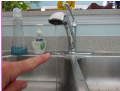
Low hot water flow at kitchen sink.
