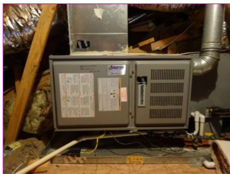
Nat Gas fired furnace located in attic.
