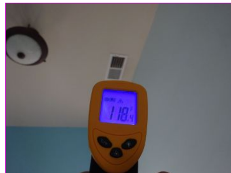
118 degrees at supply when heat was on.
