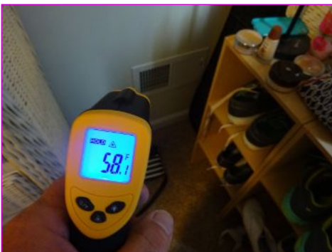
58 degrees at supply in cooling mode.
