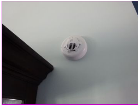
GENERAL INTERIOR Smoke/CO Detectors
