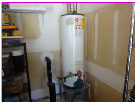
Nat. Gas Water Heater located in Garage.
