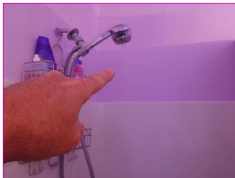
Low flow at shower while tub faucet running.
